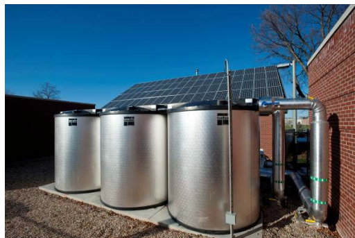
Thermal Storage Tanks & Solar Electric at the Academic Village Residence Hall
