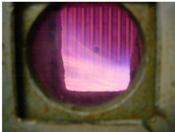
Boiler at CSU’s District Energy plant
